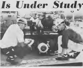
ONE OF THE first steps taken in Lago's Oil Conservation Survey was a personal inspection of hydrocarbon pumps to stop oil losses caused by leaky pumps. Checking an isobutane pump is B. W. Vignealet, left, who made the survey, and T. M. Bacon of TSD-Laboratories. UN DI e pramer panson tamá den estudio na Lago pa conservacion di azeta baltico un inspeccion personal di pompnan di hidrocarbón pa stop tur desperdicio di azeta causa door di pompnan cu ta lek. Controlando un pomp di isobutano ta B. W. Vignealet, banda robes, hace e chec e estudio, y T. M. Bacon di TSD-Laboratories.
